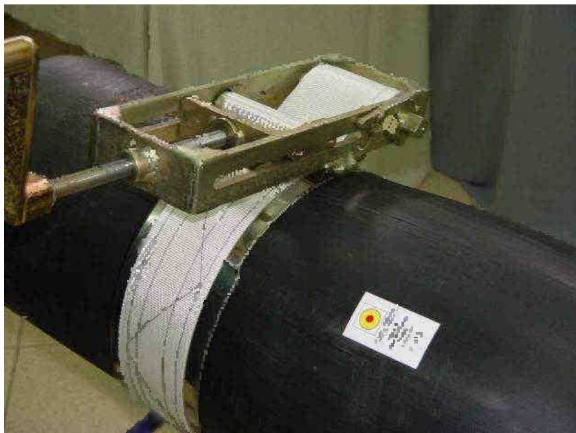
Photo 46 A view of a heat shrinkable, metal separator tightened together with a belt fastener
